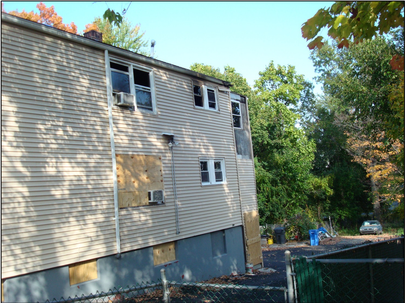
Photo 4. Side Delta of the structure. A rear entrance leads to the first- and second-floor apartments on the Delta/Charlie corner (NIOSH photo.)
