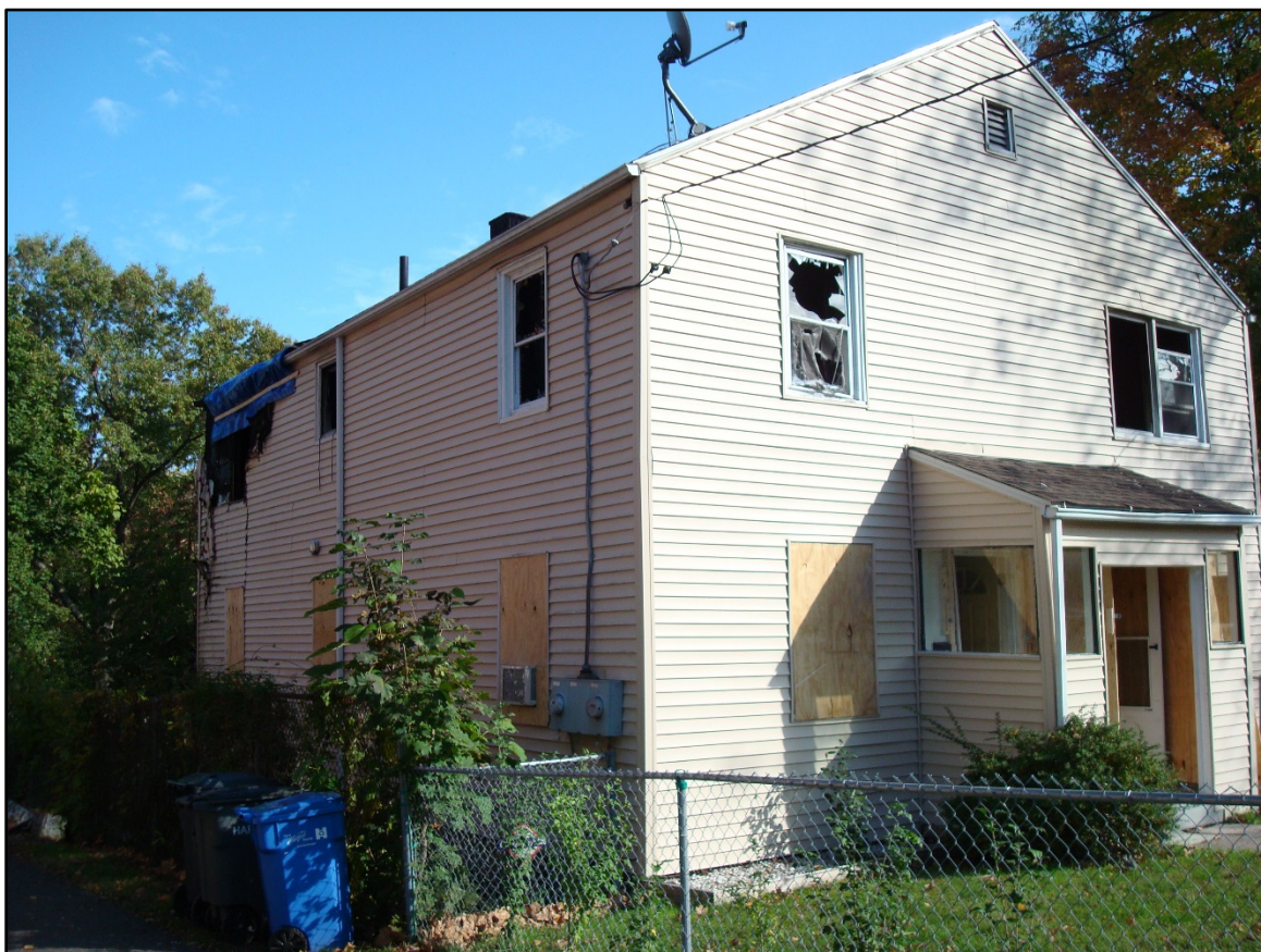
Photo 2. Side Bravo—street view of the duplex. Origin of fire near the Bravo/Charlie corner on the second floor. (NIOSH photo.)
