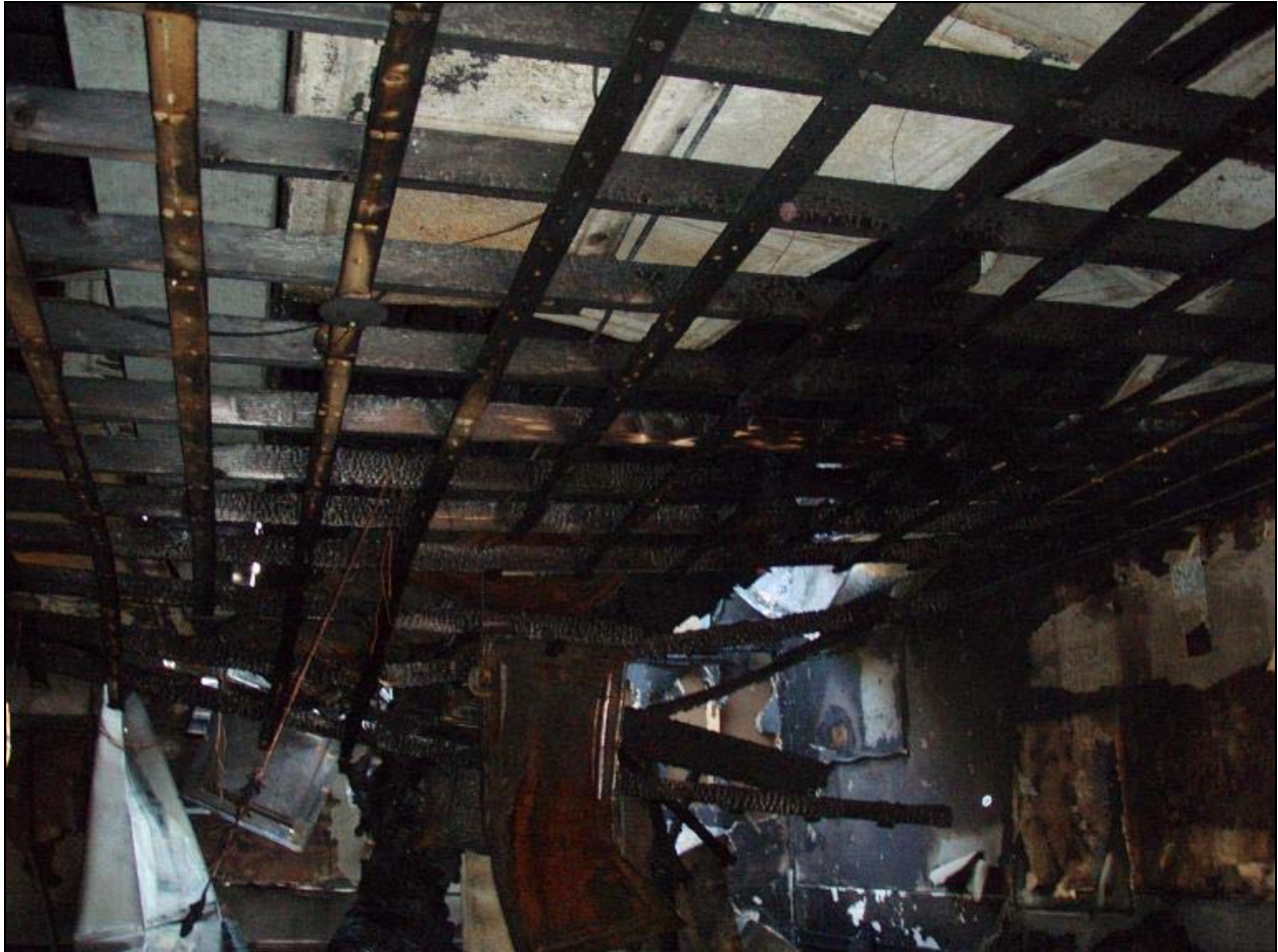
Photo 6. View looking towards kitchen and D-Side wall from dining room at exposed furring strips where the ceiling tiles were attached prior to the rapid fire event. (Photo courtesy of fire department.)
