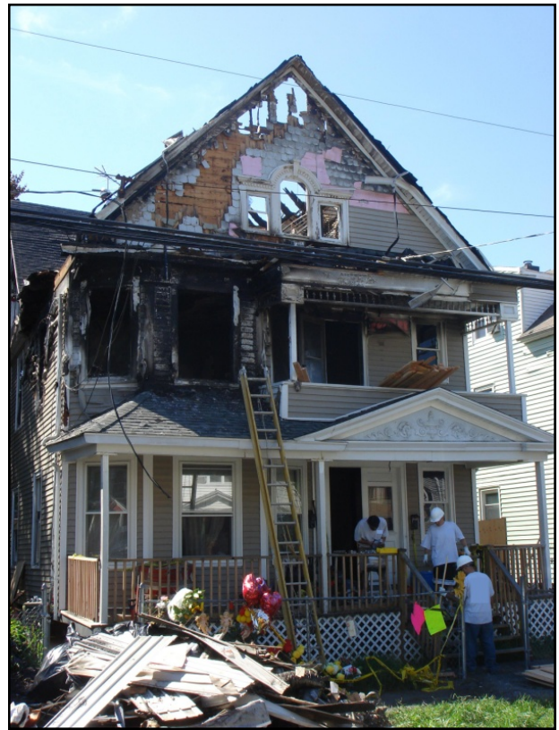
Photo 1. A-side of house during cleanup operations. (NIOSH photo.)
