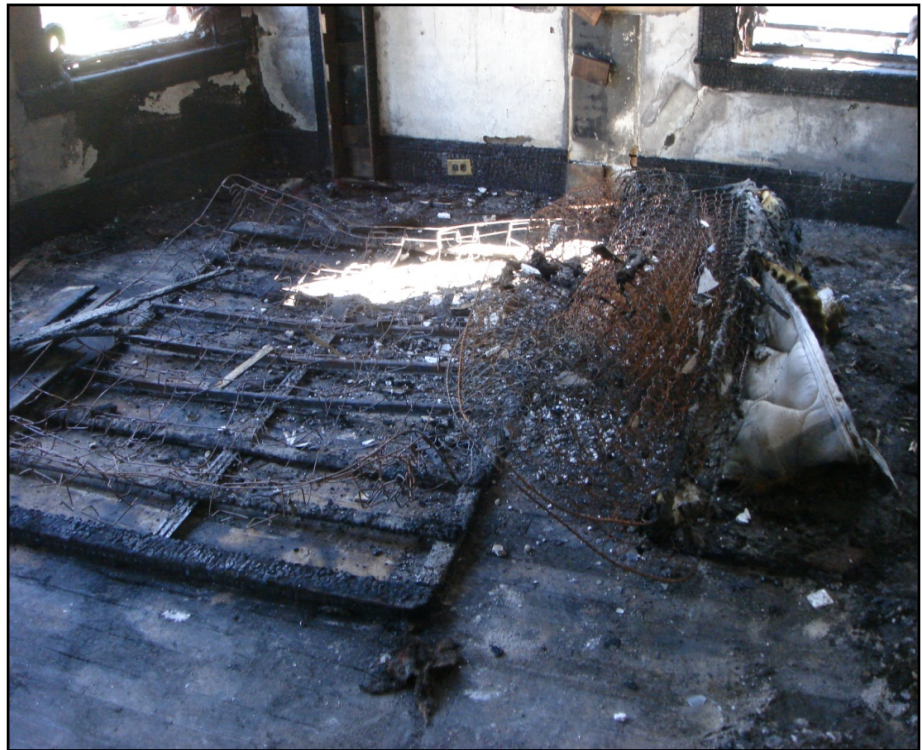
Photo 2. Remnants of a mattress and box springs within the room of origin on the 2 nd floor. (NIOSH photo.)
