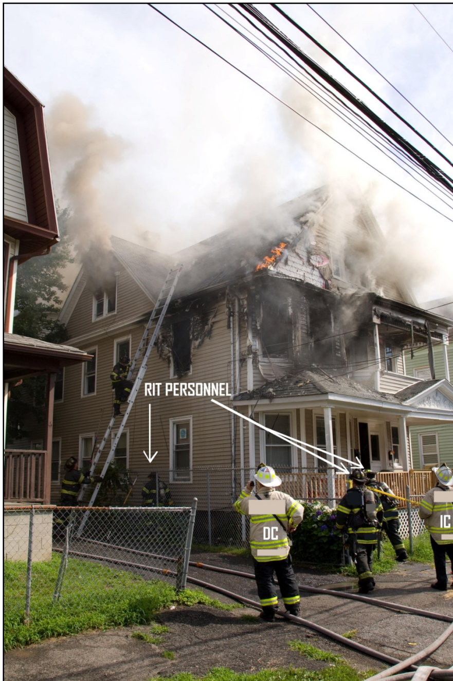
Photo 9. Mayday for Victim #1, called by FF2. Note: RIT personnel from E12 are seen heading to the rear of the house. L5 personnel were descending the roof via the B-side ground ladder. Fire is seen burning along the roof line above the A/B corner. Gray, dense smoke was flowing from the 3 rd floor B-side double window and A-side window. (Photo courtesy of Keith Muratori.)
