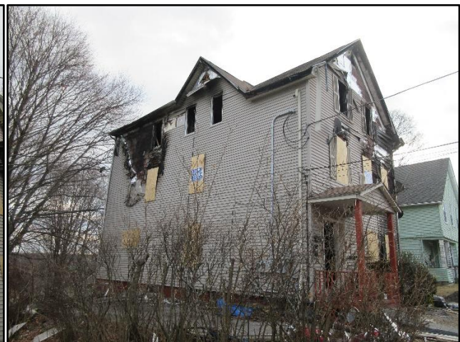
Photo 2. Side Bravo of the structure. Note the heavy fire damage from the bedroom where the fire originated. NIOSH Photo
