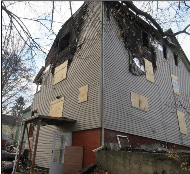
Photo 3. Side Bravo and Side Charlie of the structure. Note: The awning over the basement door was where the chauffeur of Ladder 5 landed when the lieutenant pushed him out the 3 rd floor window. NIOSH Photo
