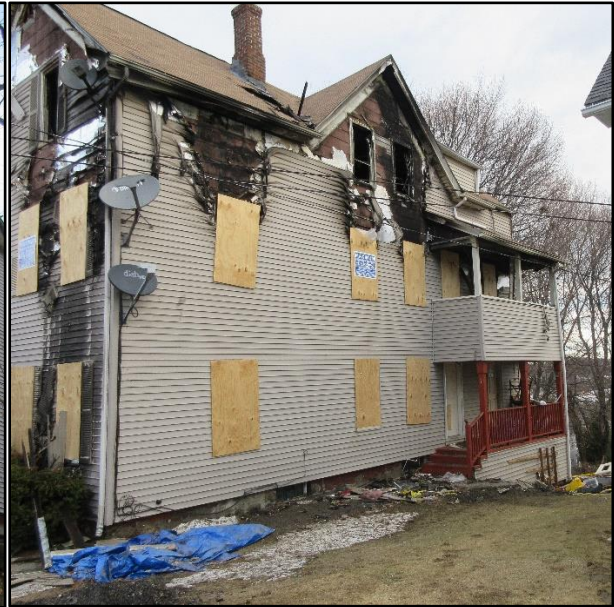
Photo 4. Side Delta of the structure. Engine 15 entered the door on Side Charlie to attack the fire on the 2 nd floor. NIOSH Photo
