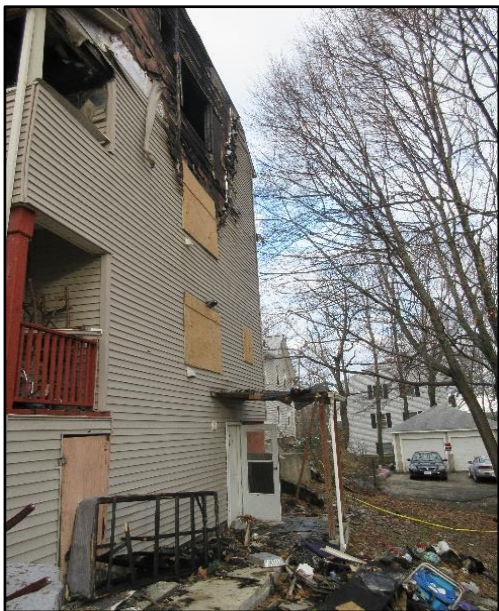
Photo 8. 3 rd floor porch window Ladder 5 firefighter went out of and initially landed on awning over basement door. NIOSH Photo
