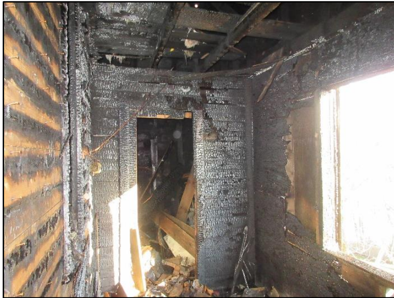
Photo 12. Third floor porch shed breached by Rescue 2 where Ladder 5 Lieutenant took shelter. NIOSH Photo
