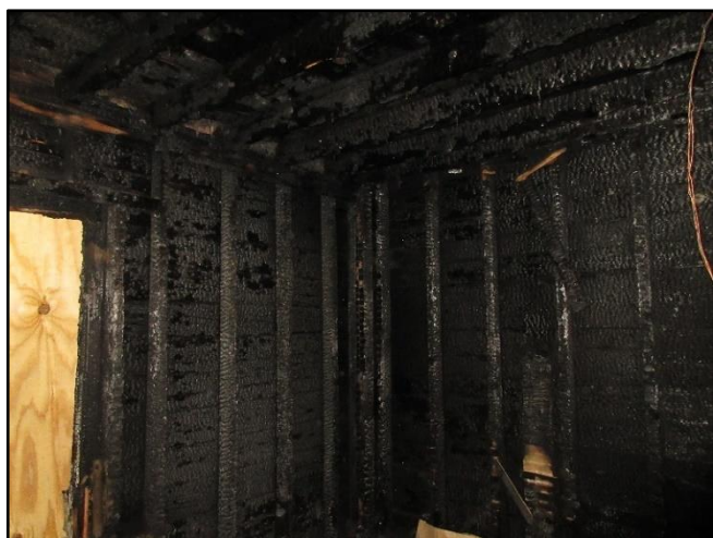
Photo 6. 2 nd floor bedroom that was on the Side Bravo/Side Charlie corner. NIOSH Photo
