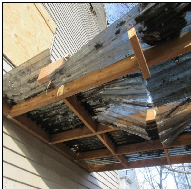
Photo 9. View of awning which reduced the impact when the Ladder 5 firefighter hit the concrete pad on the ground. NIOSH Photo
