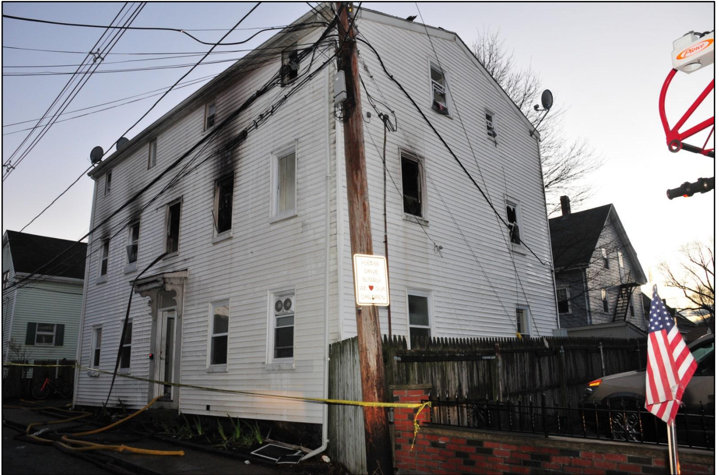
Photo 1. The apartment building viewed from the “A/D” corner. The window above the doorway is the hallway landing on the 2nd floor.
